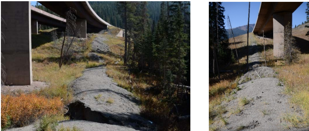
Figure 1. Side cast in bridge areas across perennial tributaries is easily transported to Black Gore Creek each year. Building access grades to these zones would allow for periodic removal.
